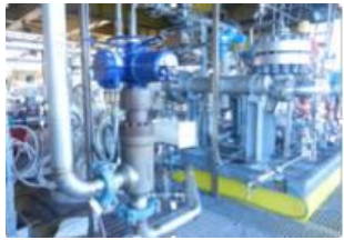
Retrofit modular water treatment cyclones (FMC Technip)
